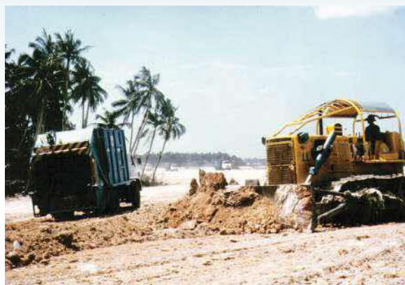
Bulldozer covering refuse with a layer of earth at the Lorong Halus Dumping Ground, late 1980s and early 1990s. Courtesy of the National Environment Agency.
