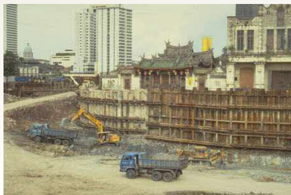
River works at Magazine Road, with Tan Si Chong Su temple, a National Monument, in the background, 1980. Ronni Pinsler Collection, courtesy of the National Archives of Singapore.
